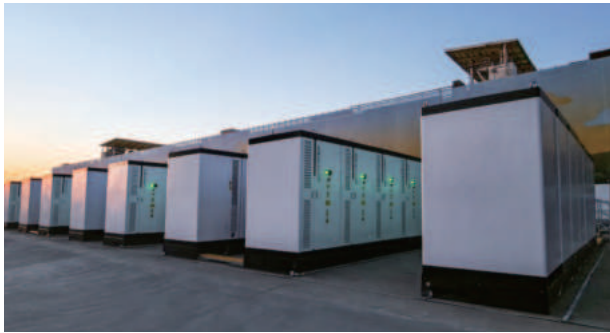
Hungary MVM Utility-scale 31MW/75MWh Energy Storage Project
