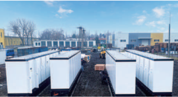
Hungary C&I 6MW/12MWh Energy Storage Project
