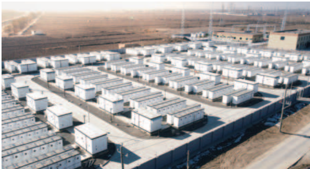
Niushoushan 200MW/400MWh Energy Storage Power Station Project
