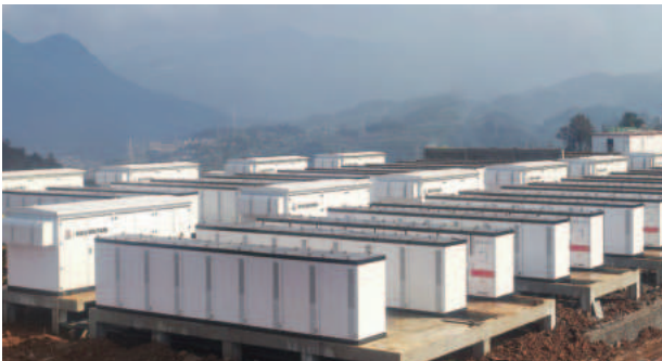
Zhendong Electrochemical 100MW/200MWh Energy Storage Project
