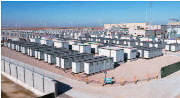
Dongying Jinhui Independent Shared 100MW/200MWh Energy Storage Project
