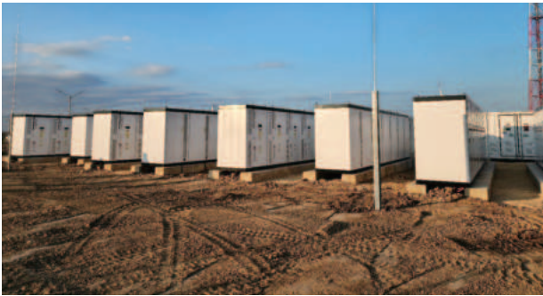
Hungary MVM Utility-scale 11MW/22MWh Energy Storage Project
