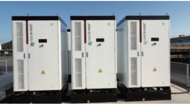
Japan C&I 1.29MW/2.508 MWh Energy Storage Project
