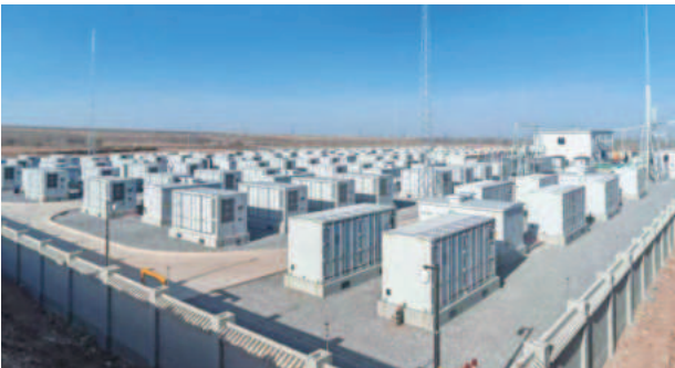
Ningxia Hanjun 150MW/600MWh Energy Storage Project
