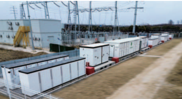
Tongwei Yancheng 10MW/20MWh Energy Storage Station
