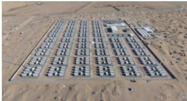
Inner Mongolia Dengkou 500MW/2000MWh Energy Storage Project
