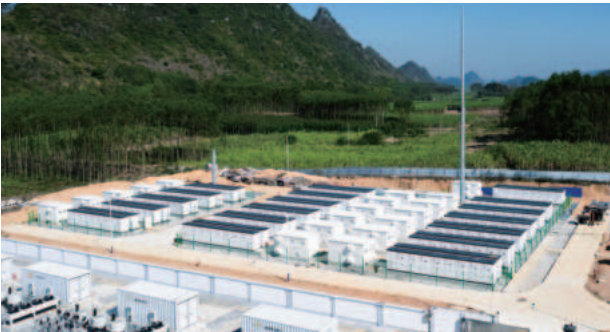
Guangxi Guigang 144MW/288MWh Energy Storage Station Project
