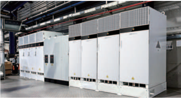
Germany Oldenburg C&I 2MW/4MWh Energy Storage Project
