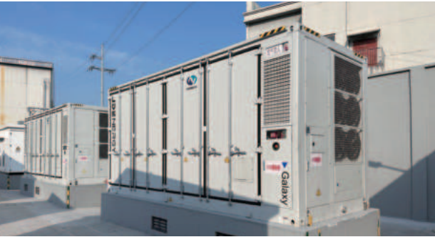
Hengyi Petrochemical 33.5MW/67MWh Energy Storage Project
